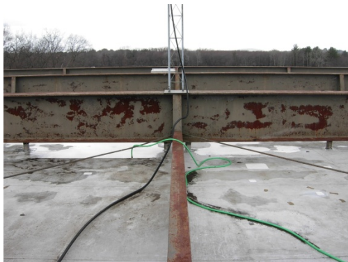
Deteriorating steel structure
