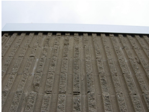
Strong winds have entered between fluted block and flashing and lifted the EPDM off of the roof
