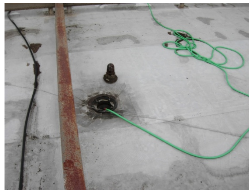
Failing roof drains and thermal bridging of exposed structural steel
