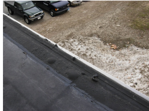
EPDM blistering and failing roofing adhesives.
